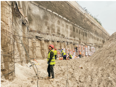
(a) 某砂层基坑桩间流砂
