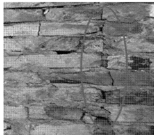
(c) 墙体裂缝
