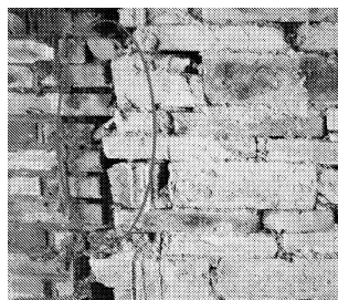
(a) 墙体无可靠搭接
